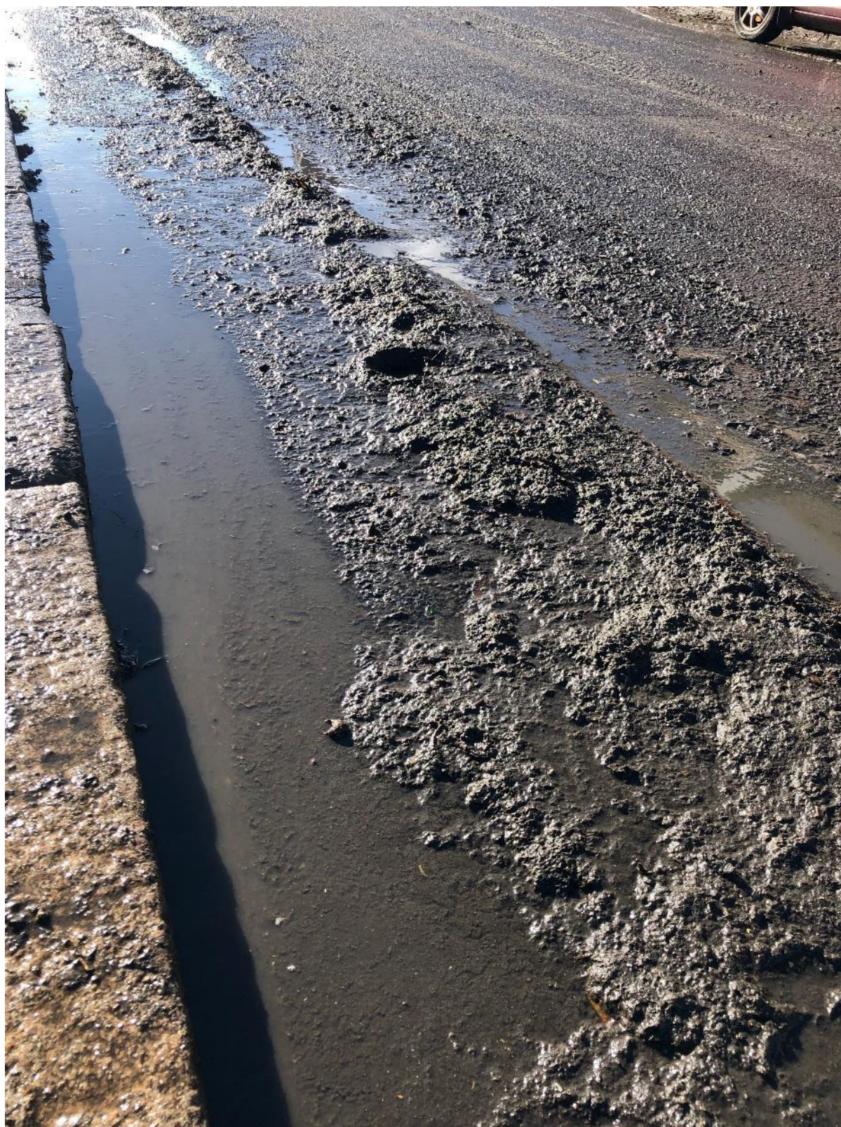
Photo 5: Post flooding debris (1)
