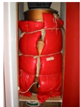
Poorly insulated and badly fitted
