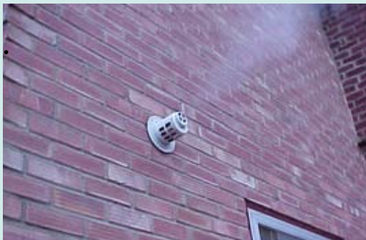
A pluming boiler flue
