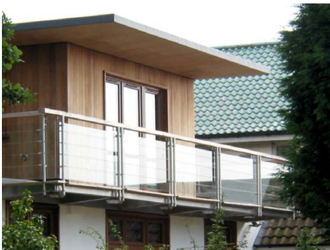
Good quality materials and detailing on a rear extension in Eastwood Road.
